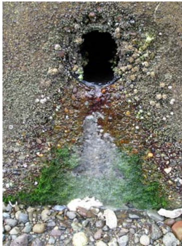
OSS effluent flowing out of a Bulkhead Drain into Hood Canal
