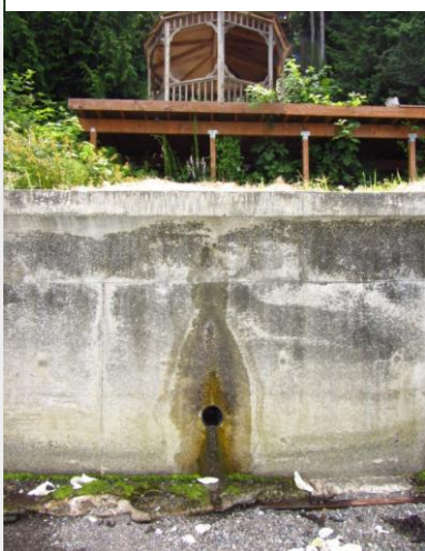
Photo 5 Bulkhead Drain Monitoring Location
