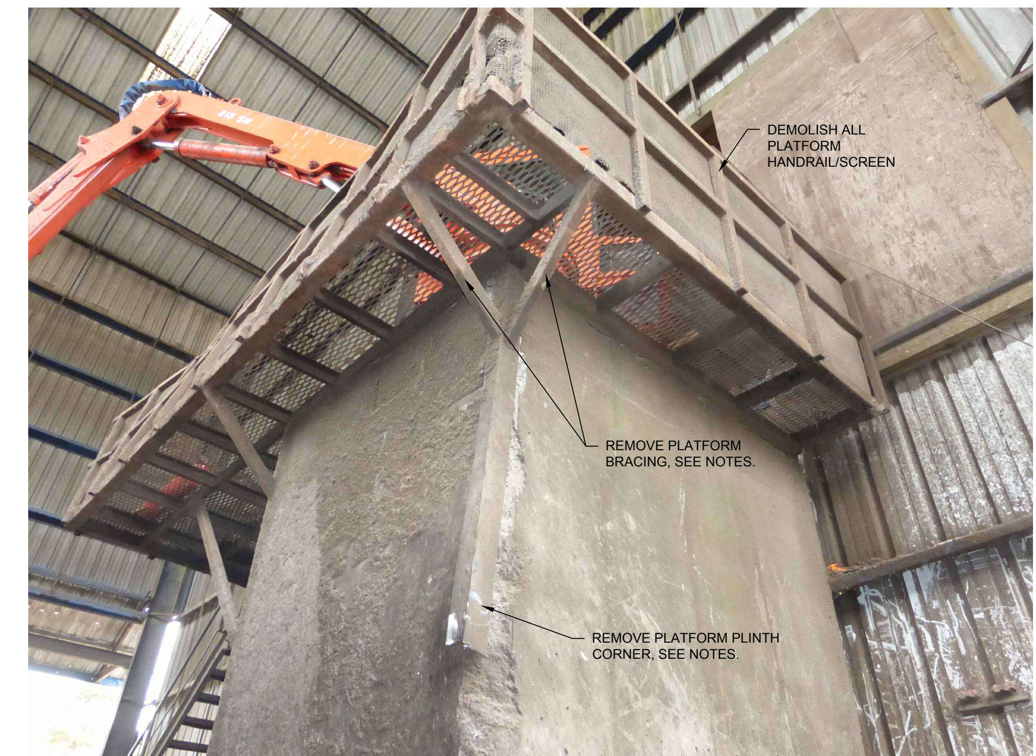
SEE 6 S-007 PLATFORM BRACE AND PLINTH CORNER EMBED REPLACEMENT 1 - N.T.S. CRANE PLATFORM DEMOLITION DETAIL
